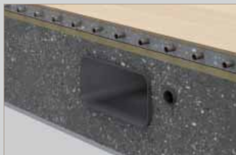
Shallow duct in the reinforced concrete floor
